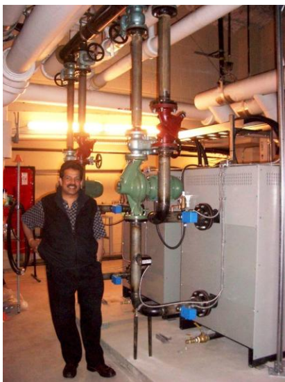
Priyan Jayetileke with the Sempa Hybrid Heating System at Four Seasons Whistler
